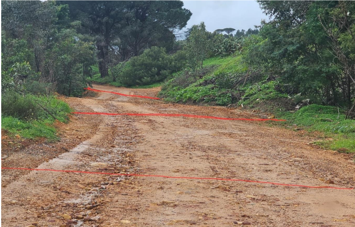
Figure 9.) Drainage on existing road during heavy rainfall -current (actual)
