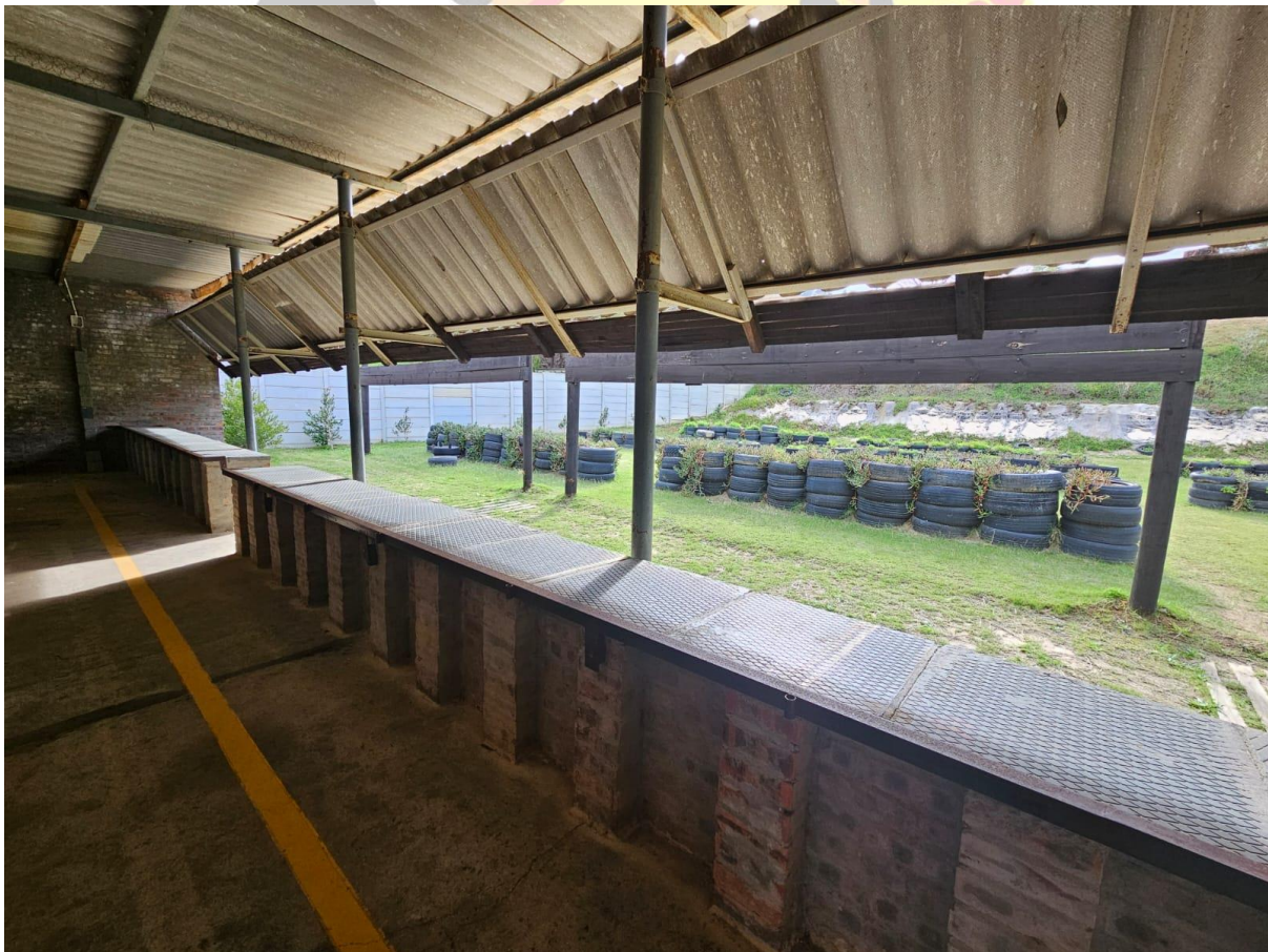
Figure 7.) Main range- note tyre walls, preformed concrete deflections walls and Carpobrotus spp (actual)
