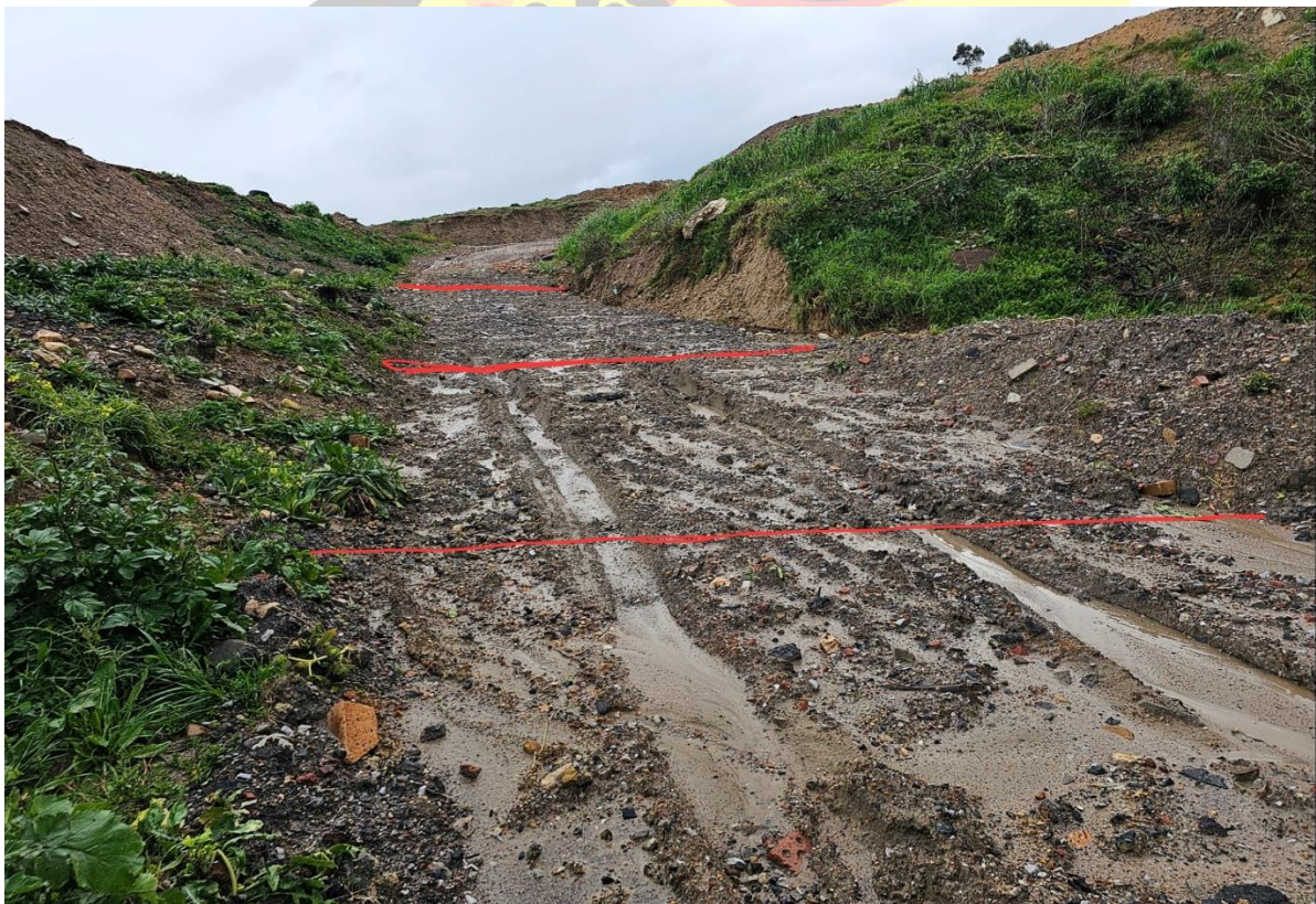
Figure 8.) Drainage on existing road during heavy rainfall -current (actual)
